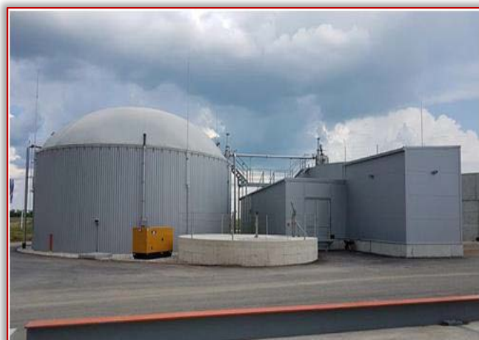
Figure 4. Biogas power plant (300 kW) in the Hrastin village
