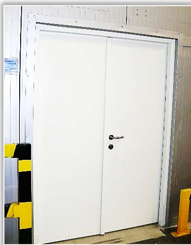
Figure 5. Acoustic entrance door
