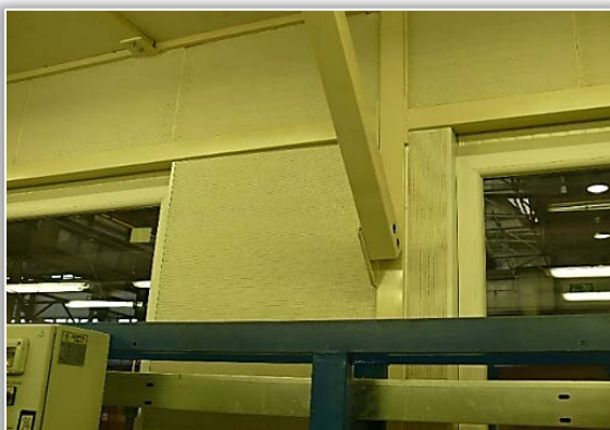
Figure 6. Installed sound absorption materials
