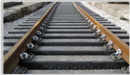
Figure 16. Plastic composite railroad ties
