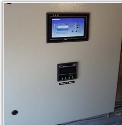
Figure 2. PLC with electrical cabinet
