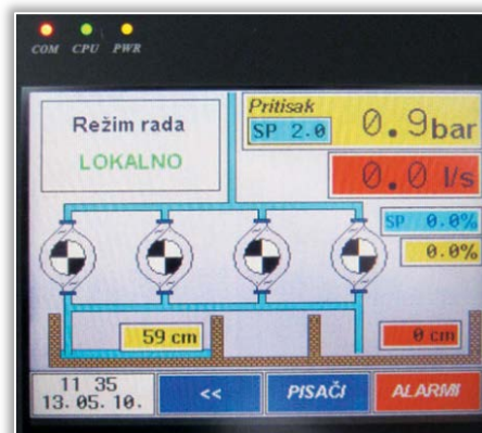
Figure 1. Remote control panel for process automation
