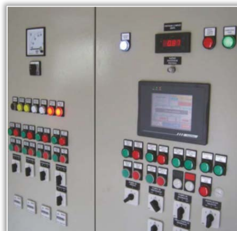
Figure 3. Electrical cabinet with touch screen panels
