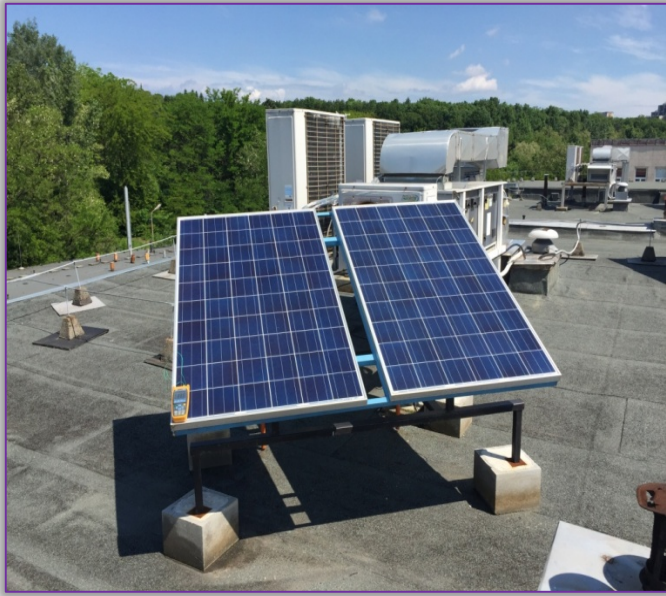
Figure 3 -Solar panels used for the measurement
