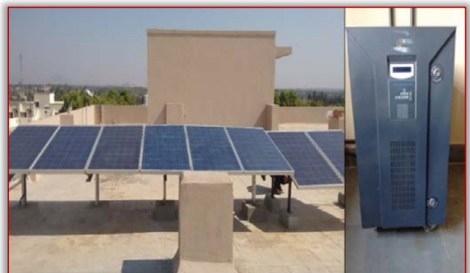
Figure 3. Solar PV panels with inverter
