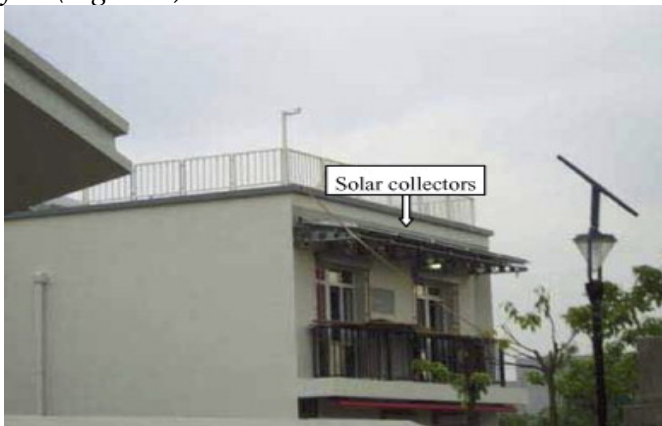
Figure 3. Solar hot-water system in villa
