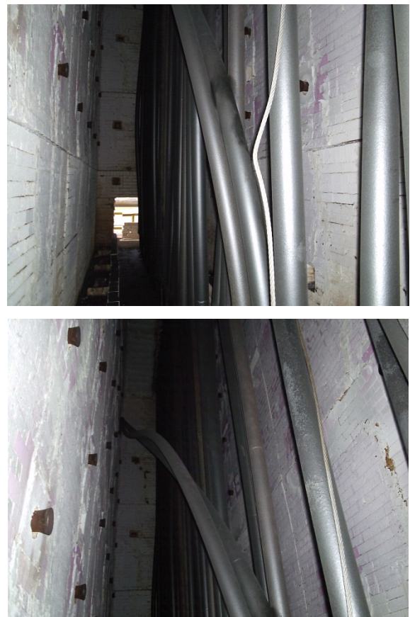
Figure 2. Pyrolysis furnace radiant zone - consequence of a high creep rate
