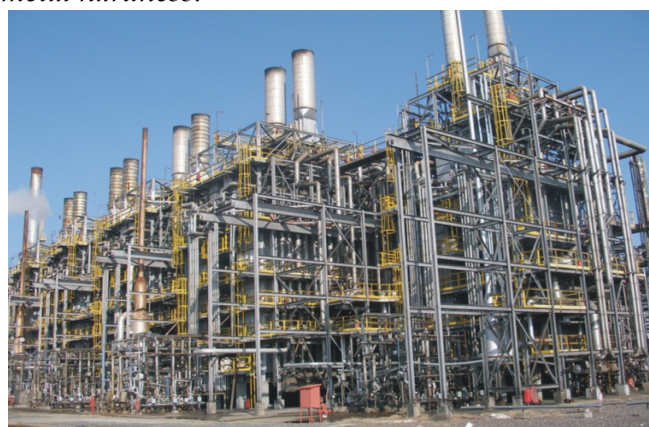
Figure 1. Pyrolysis furnaces in ethylene plant
