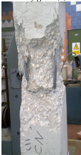
Figure(4) Failure mode of column (Experimental)
