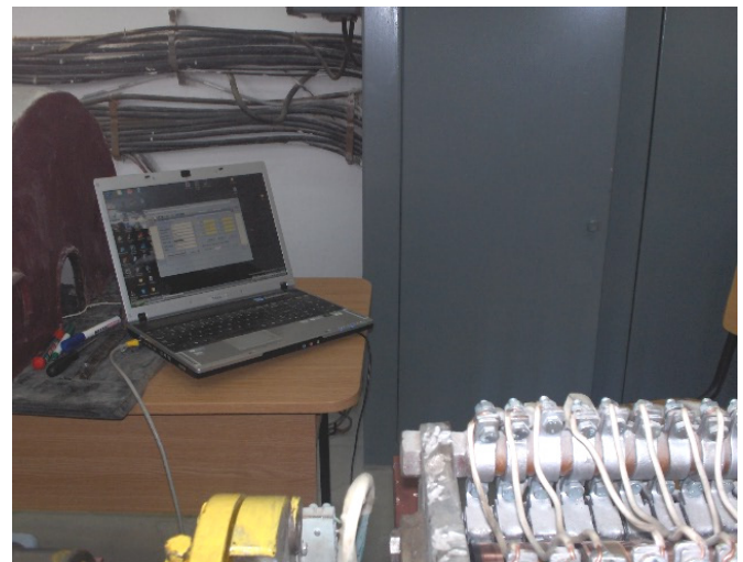
Figure 11. The connection to a data acquisition system
