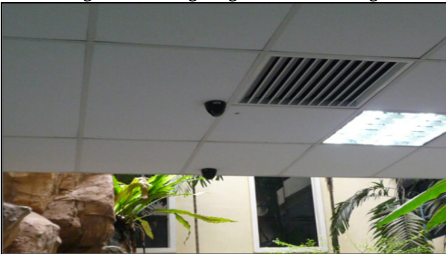
Figure 7: Speed dome at ground floor in Eureka building
