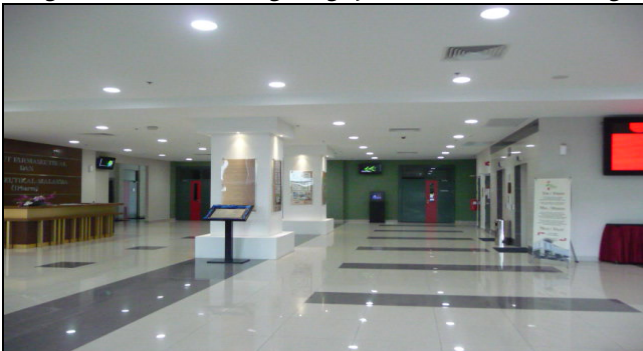
Figure 6: Cove lighting in IPharm building
