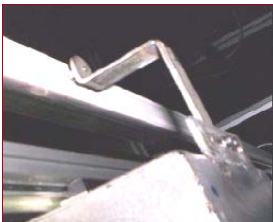
Figure 7: Scanning of the position of elevator cabin with means of a magnet moving along the sensor plinth
