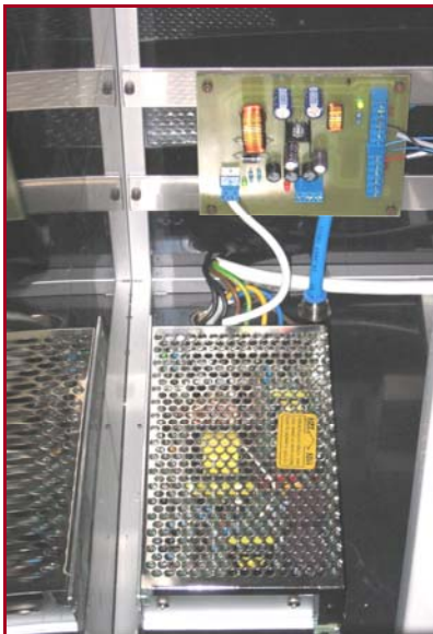
Figure 6: Realization of power supply of the elevator
