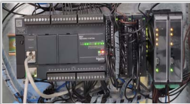
Figure 3. PLC Schneider Electric M221 with analog input/output modules and the proportional controllers located in the electrical cabinet
