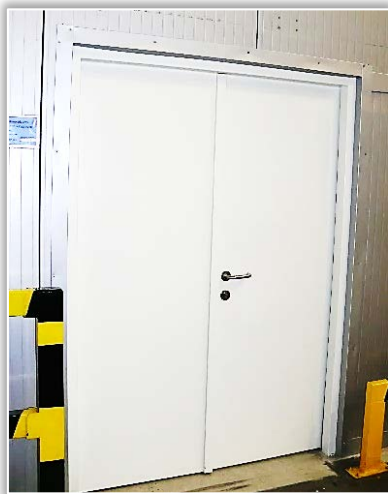
Figure 5. Acoustic entrance door
