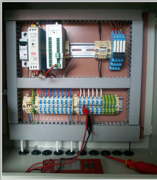
Figure 8. Electrical cabinet with a GPRS modem
