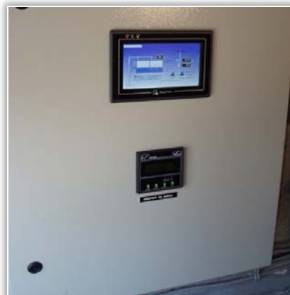
Figure 2. PLC with electrical cabinet
