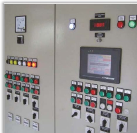
Figure 3. Electrical cabinet with touch screen panels
