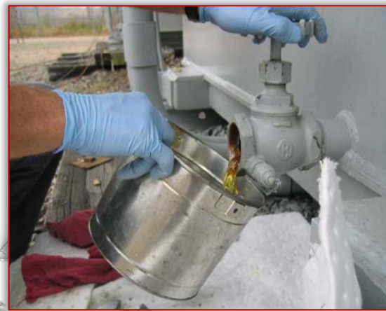
Figure 3: Discharge of oil at the lowest point of transformer
