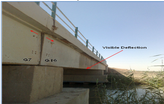
Figure 5. Visible mid span deflection at the right side of the intermediate panel
