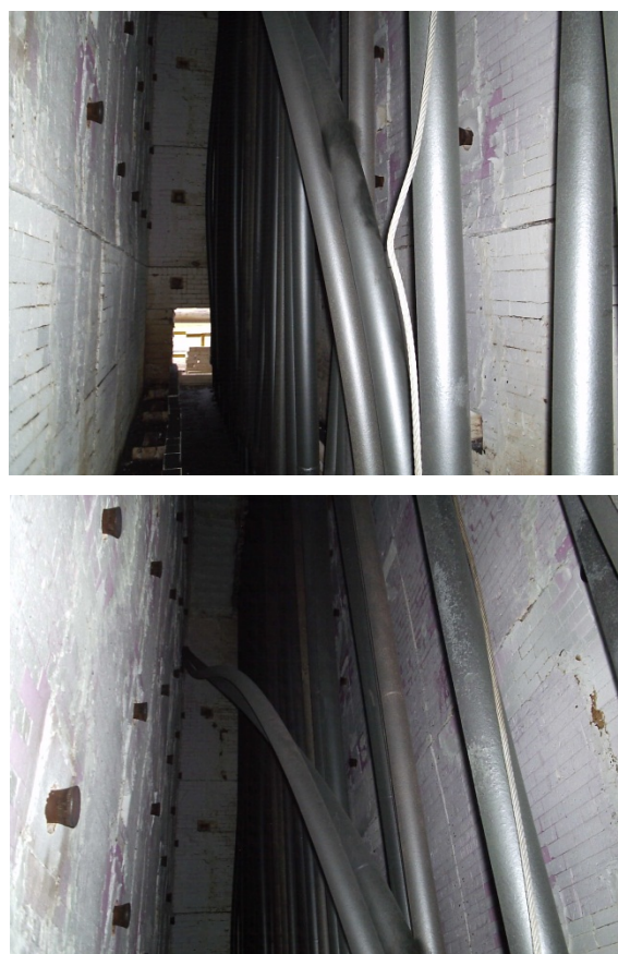
Figure 2. Pyrolysis furnace radiant zone - consequence of a high creep rate
