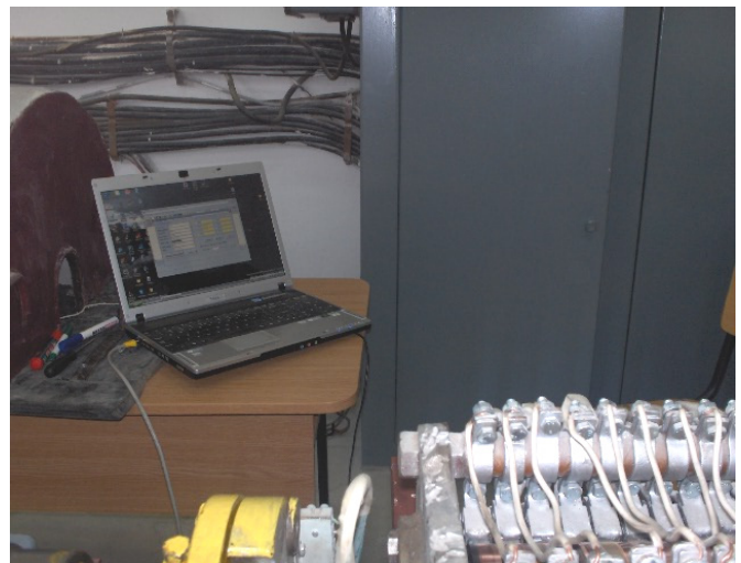
Figure 11. The connection to a data acquisition system
