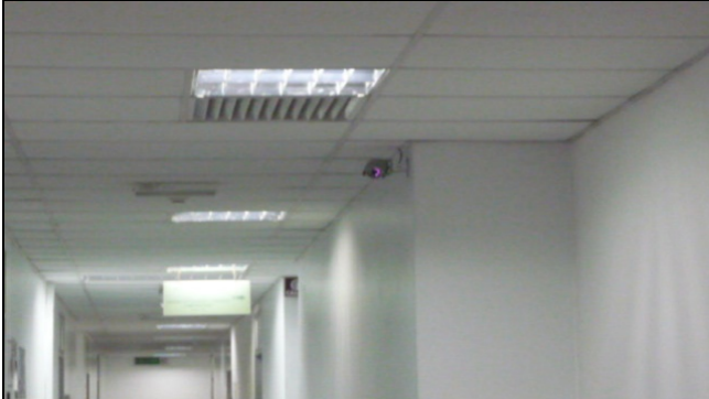
Figure 5: Fluorescent lighting system in Eureka building
